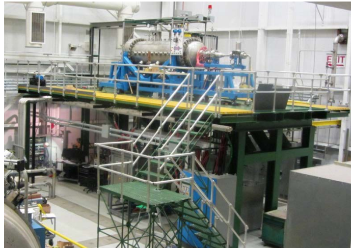
NTREES Phase 2 – 1MW Upgrade (2015)
